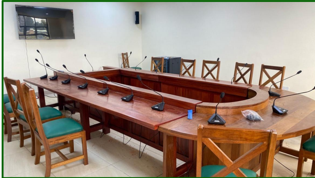
Hansard Equipment installed in Committee rooms
